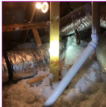
Ductwork laying on the floor. This could cause condensation between the duct and the insulation. The ducts need to be hung from the rafters straps every 2 to 4 feet.
